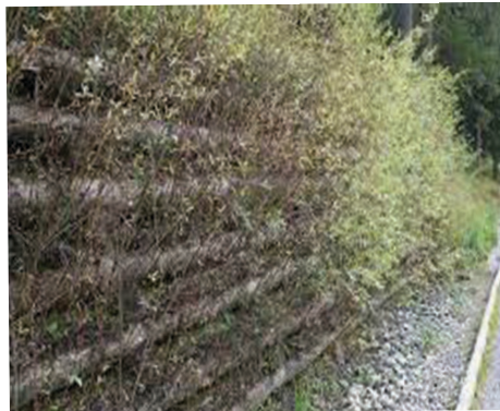
A timber crib wall uses wood posts to form a structure that is interplanted with native plants.
